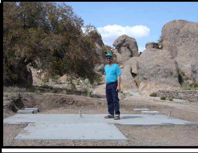
NPO President John Gilkison stands on the new City of Rocks State Park observatory pad which had just been poured prior to the Spring SNMSP
